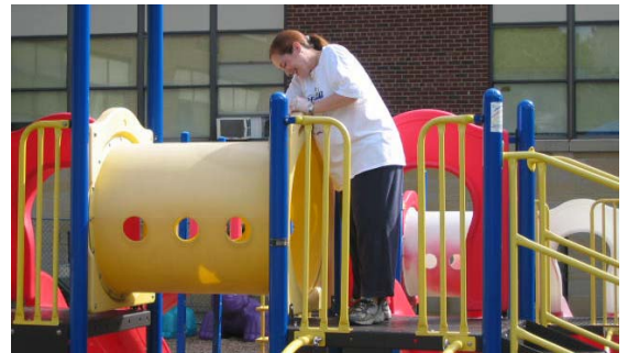
A volunteer from the Endicott Interconnect-Huron group refurbishes playground equipment at the Family Enrichment Network facility in Johnson City during the Day of Caring.
